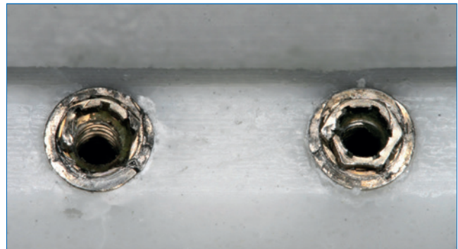
Figure 20. Damage observed, part by part, on the experimental model: implants (completed SCLT).
